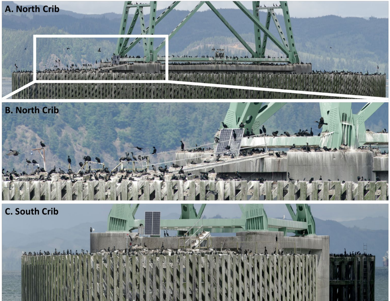
Figure 4. North crib (panels A and B) and south crib (panel C) of the Astoria Megler-Bridge from a shore-based survey on May 19, 2021.
